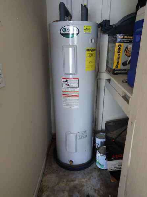
Water heater in garage
