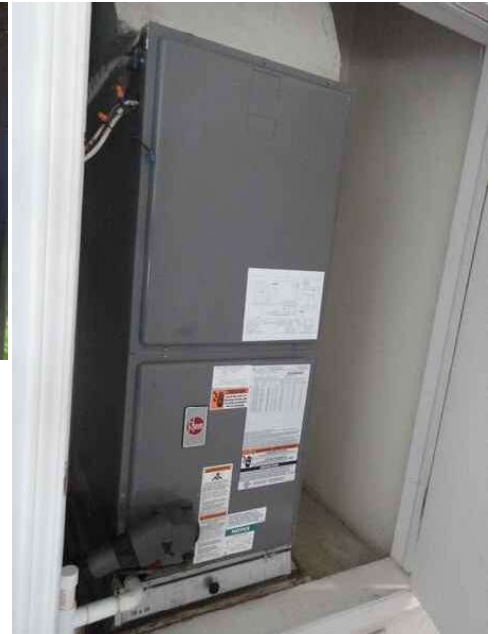
Air handling unit
