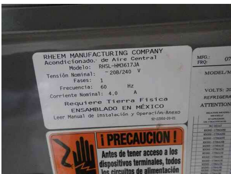
Air handling unit name plate data
