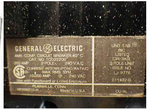
Main breaker data
