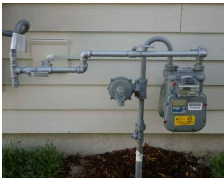
Gas meter feeding water heater and gas appliances
