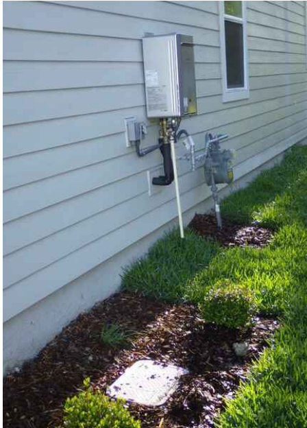
External on-demand gas and electric water heater
