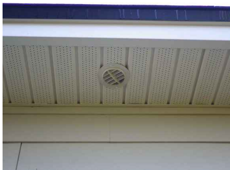
Continuous vent soffit
