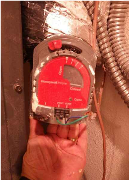
Exhaust fan in air handler closet
