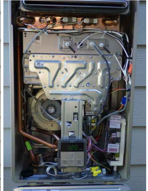
Water heater with cover off
