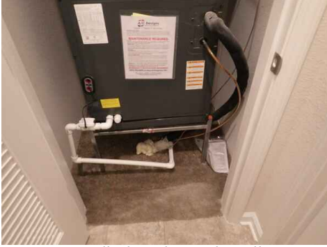
Carpet installed under air handler.
