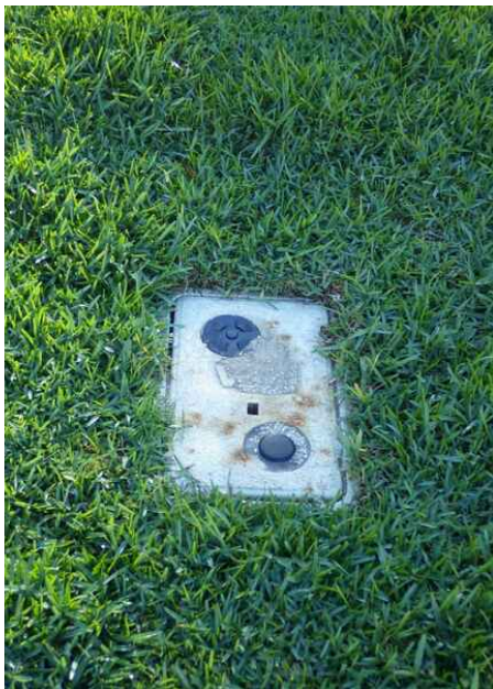
Water meter box
