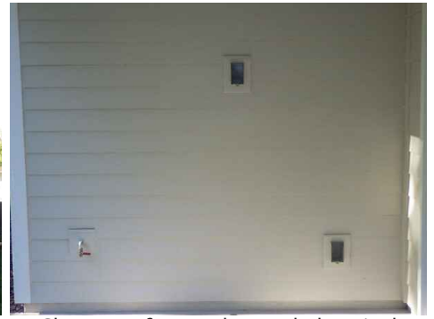
Closeup of gas valve and electrical outlets on the back porch.
