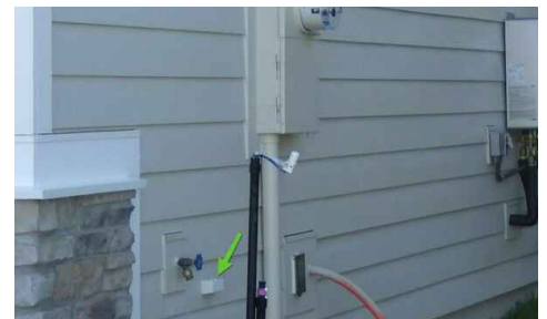
Ground wire inside wall mounted grounding appliance
