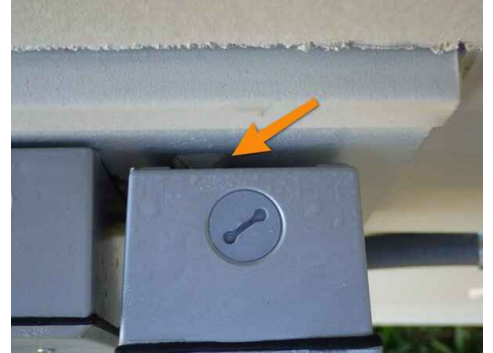
Fastener pulling out of the support block.
