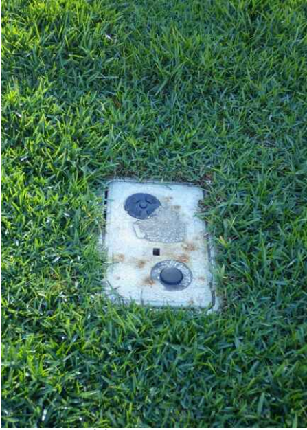
Public water meter
