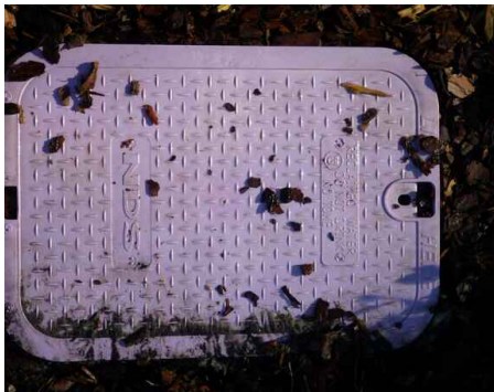
Recycled water for sprinkler system shutoff
