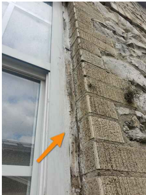
Same window, caulking defective
