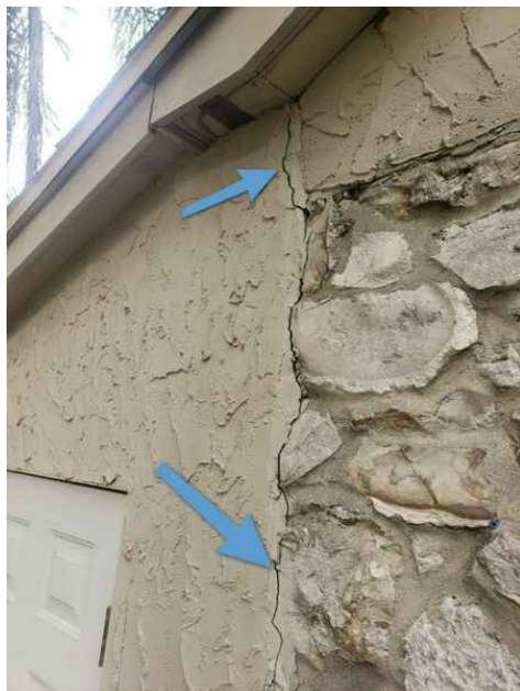
This is crack does not appear to be a structural defect however, it should be monitored as with the others, driving rain could cause water damage behind the exterior wall covering.
