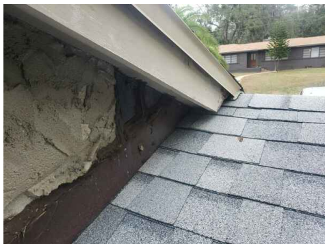
Flashing: Rubber Caulk also protecting building envelop where stucco is missing.
