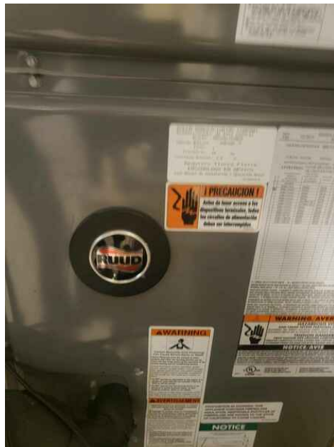
Air handling unit servicing lower level
