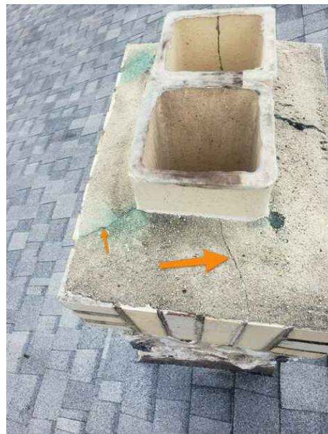
Second chimney (out of service)
