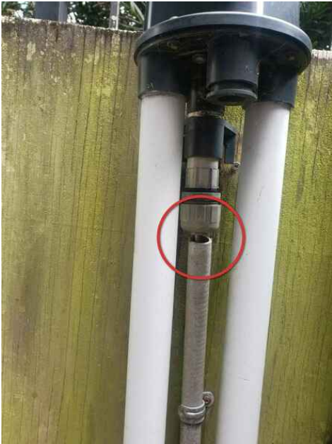
Waterproof conduit separation on outdoor connection in pool mechanical area
