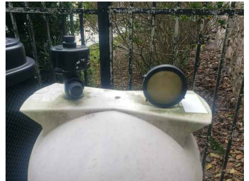
Glass cloudy and needle appears to be missing
