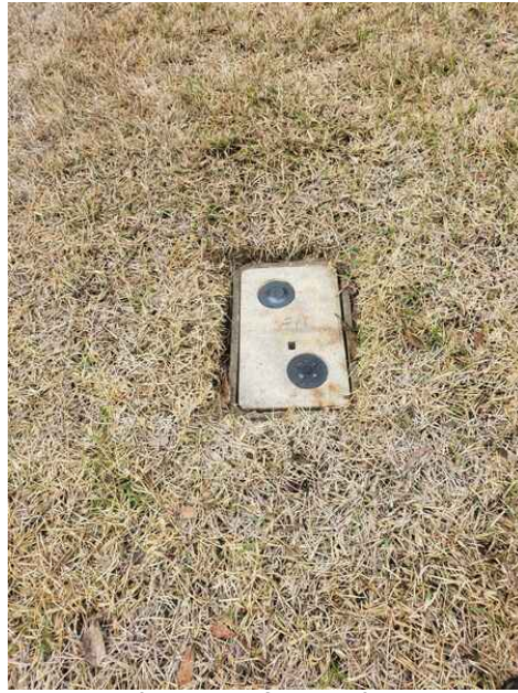
Close-up of meter box
