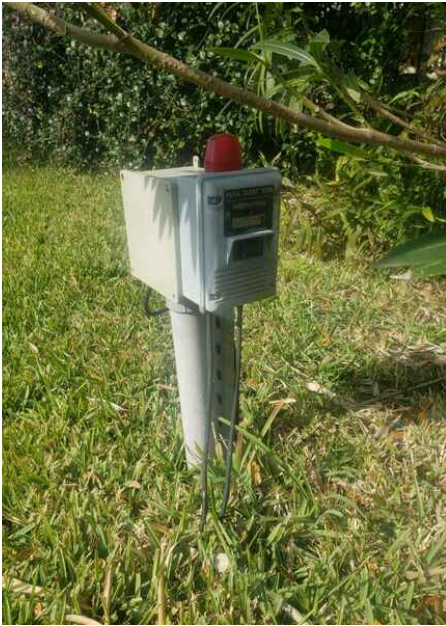
Septic Tank Warning
