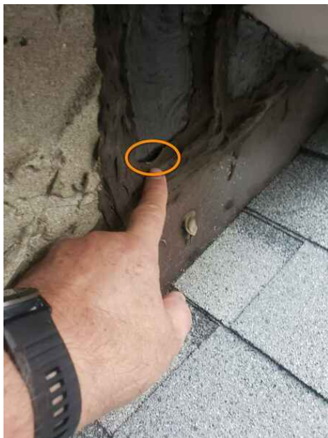
Flashing: Rubber Caulking Pulling Away
