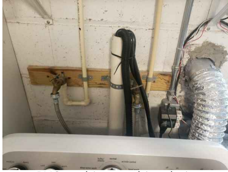
PVC washing machine drain
