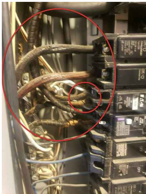
Cloth wire and double tapped wire in breaker
