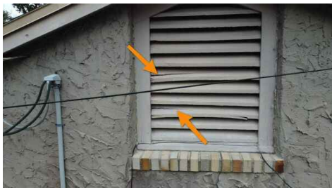
(North Gable) Louver damage visible on two boards
