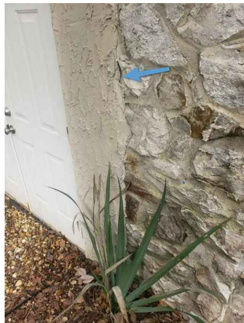
Stucco and stone lacks positive seal.
