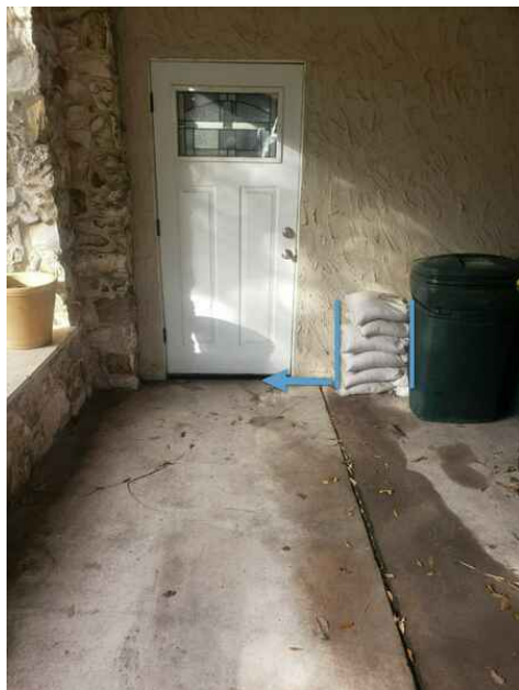
Sandbags available to block water during heavy rainfall
