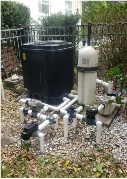
Combination of manual and electrical valves.
