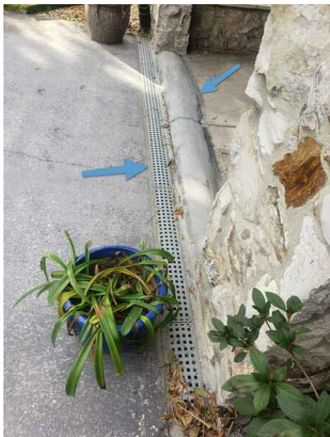
Drain and curb designed to keep water away from home.
