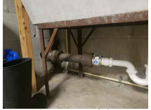
PVC to cast iron sink drain
