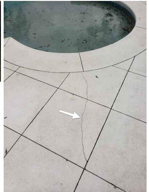
expansion and contraction crack
