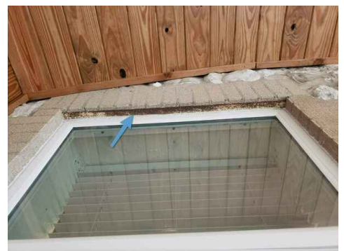
Lintel Rust (front porch)
