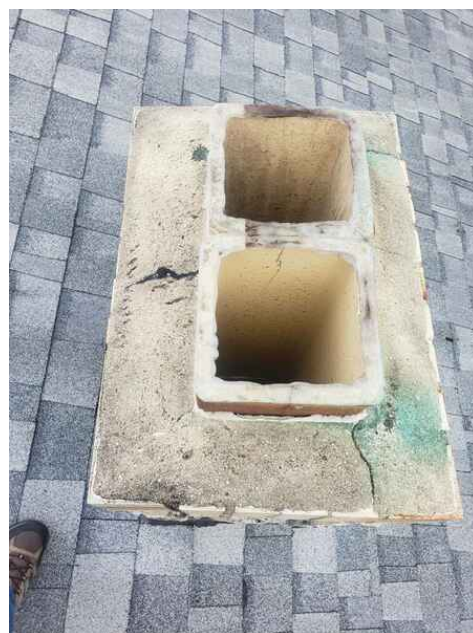
Recommend capping out of use chimney
