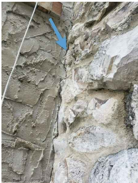
Crack where stone meets stucco. Water could pernitrate the gap and cause damage in driving rain conditions.
