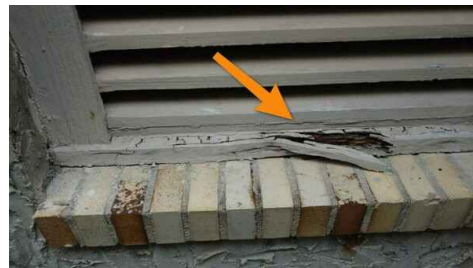
Wood rot (South Gable)
