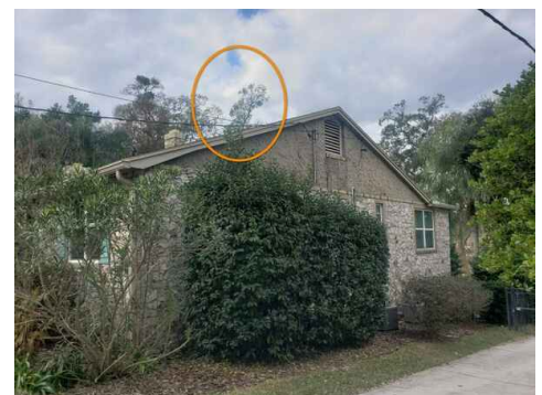
Tree growing too close to home and power line
