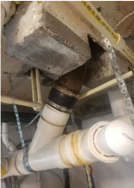
Cast iron to PVC main drain
