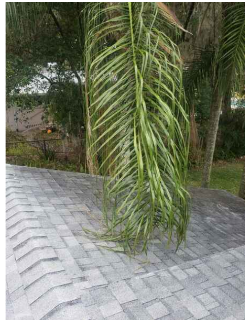
Tree touching roof
