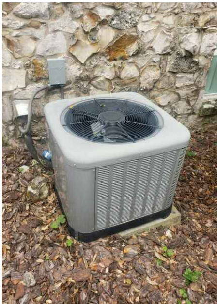
Condensing unit servicing lower floor
